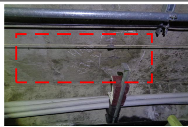
0K478 상부슬래브 균열부누수(c)(0.25m×1.0m)
