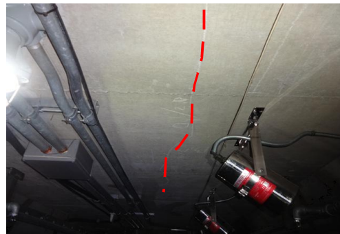
Sta.920~940m Type ① 균열 0.1/2.0
