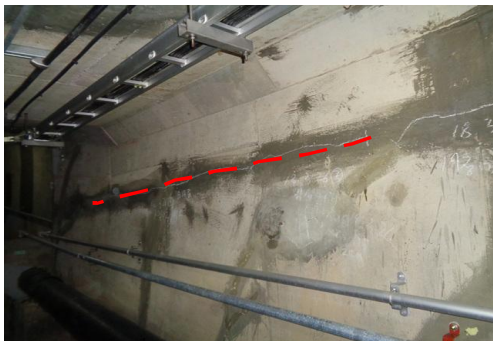
Sta.760~780m Type ② 균열 0.1/5.8
